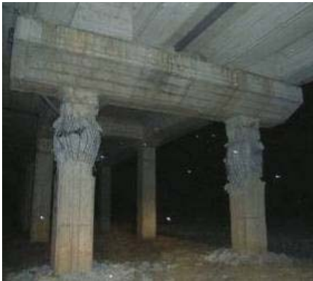
Photo 1 Damaged columns of rigid-frame viaduct
