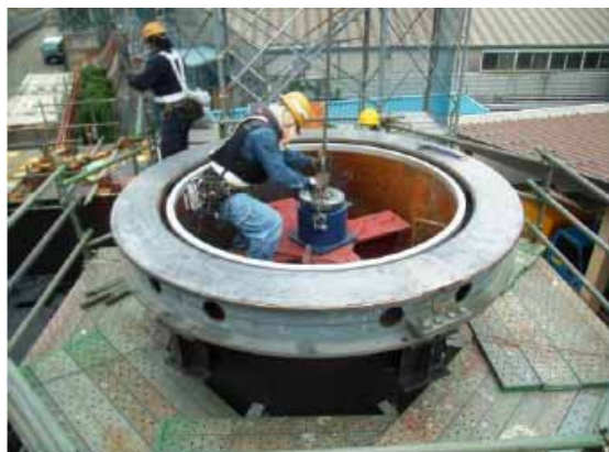
Rotation device on the top of the pillar
