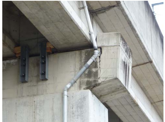
Matsuzuka Viaduct Damaged girder support (close-up)
