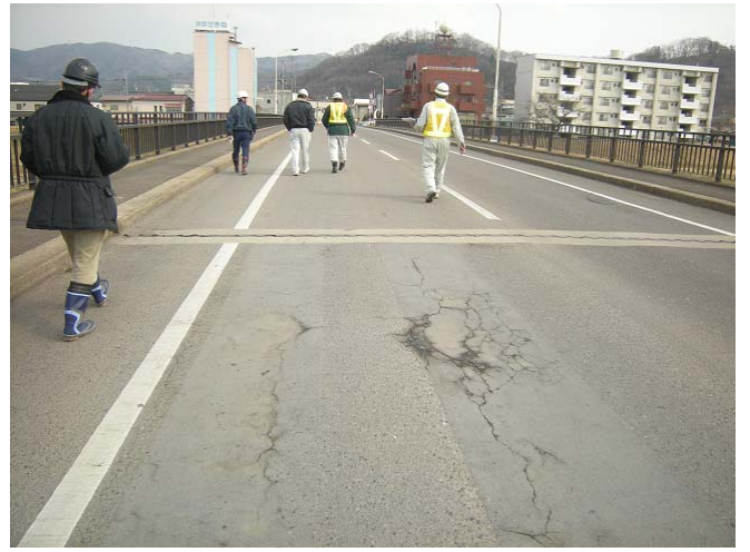
Tenjin Bbridge Bridge deck surface Cracks were observed
