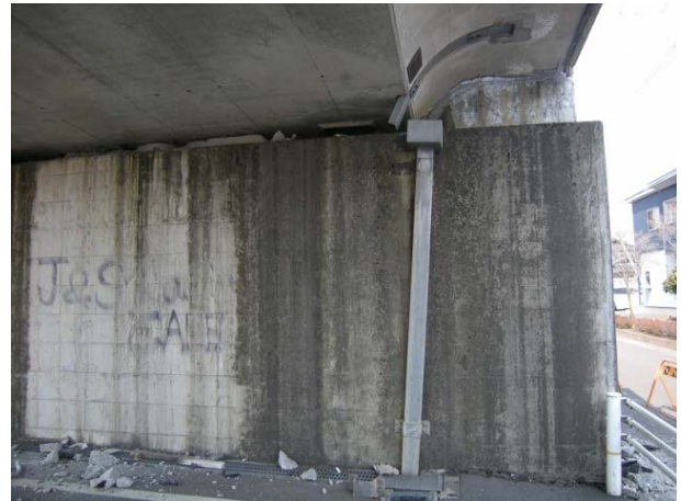
Kasaishi Viaduct A2 Damaged displacement control mechanism (anchor bar damage and fallen concrete base
