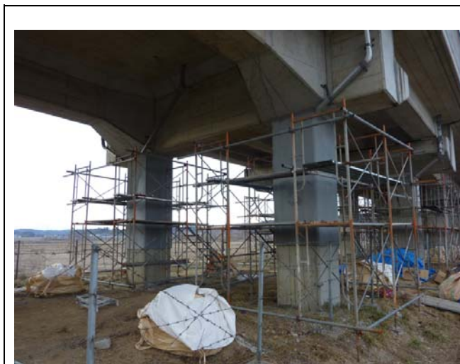
No. 2 Shijiyudan Viaduct Damaged columns being repaired by restoration of their full cross-sectional area
