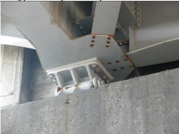
Daikokubashi Bridge Joint between P2 and G2 Severed rivets
