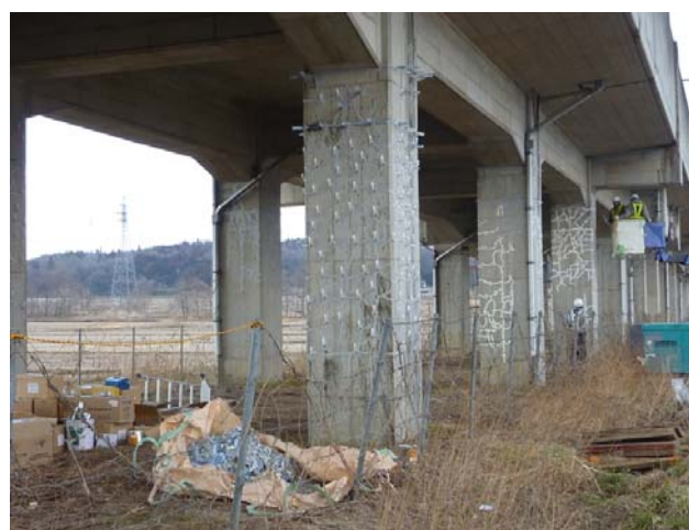
No. 2 Shijiyudan Viaduct Damaged columns being repaired by grouting the cracks with resin
