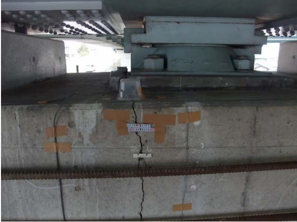
Kamedaohashi Bridge P5 on down side (steel bearing) Vertical cracks developed from the end of the steel bearing (maximum width: 11 mm)
