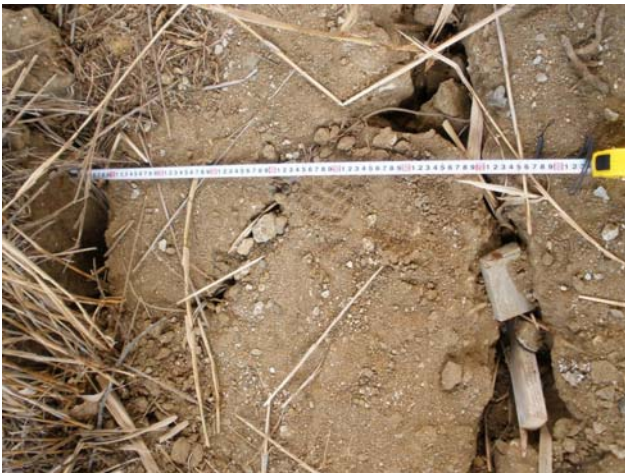
Koya Viaduct Cracks in ground at base of viaduct pier
