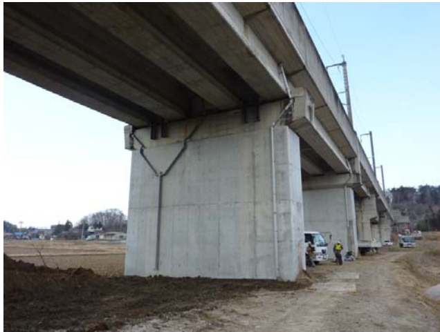
Matsuzuka Viaduct Damaged girder support
