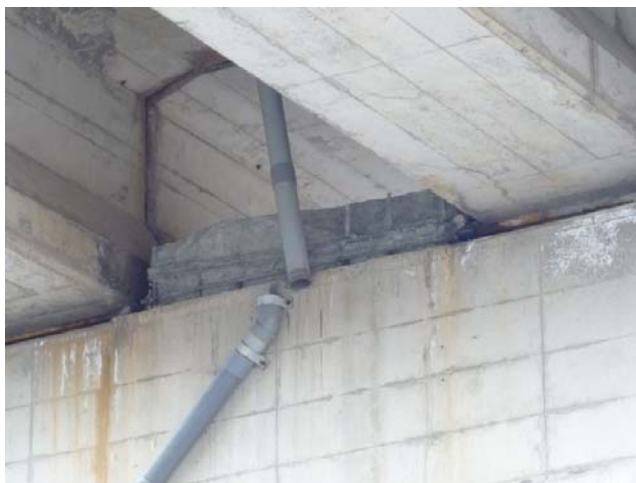
Matsuzuka Viaduct Damaged RC stopper designed to prevent falling of the girder
