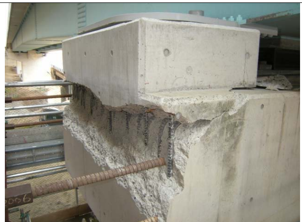
Kamedaohashi Bridge P5 on up side (RC stopper) Damage around stopper block
