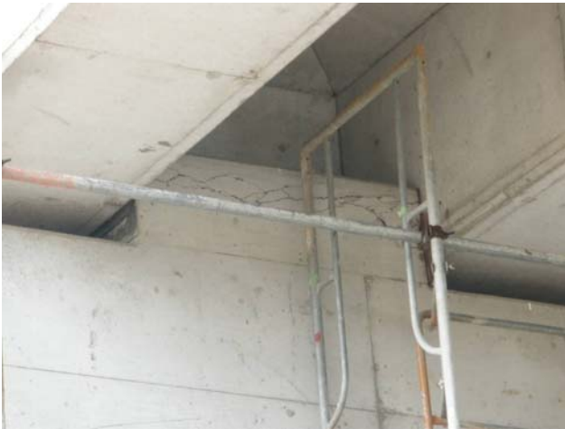
Koya Viaduct Damage to RC stopper designed to prevent falling of the girder
