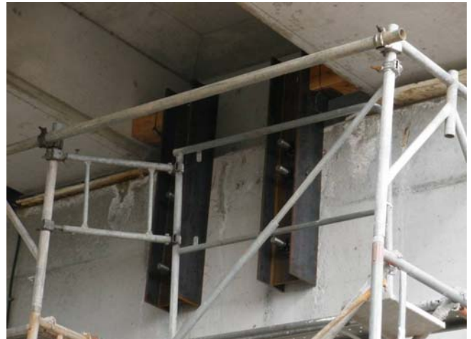
Koya Viaduct Repairs to steel restrictor shoe
