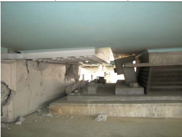
Kamedaohashi Bridge P5 on up side (rubber bearing and RC stopper) Deformed rubber bearing and damaged RC stopper
