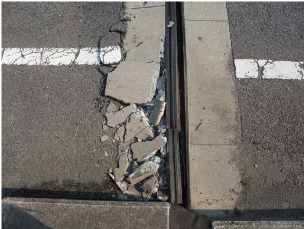
Kasaishi Viaduct Above P4 Horizontal residual displacement of girders (about 5 cm) and damaged expansion joint
