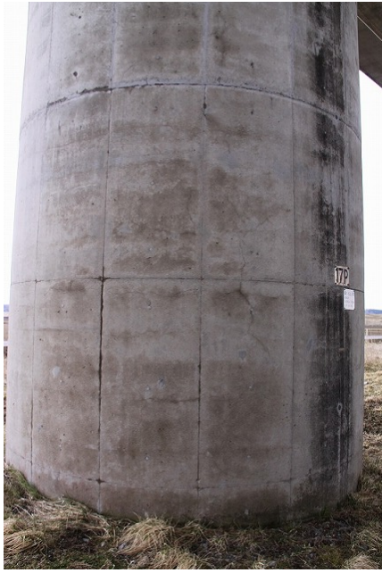
No. 1 Kitakamigawa Bridge 17 P: Minor cracks near the welded place
