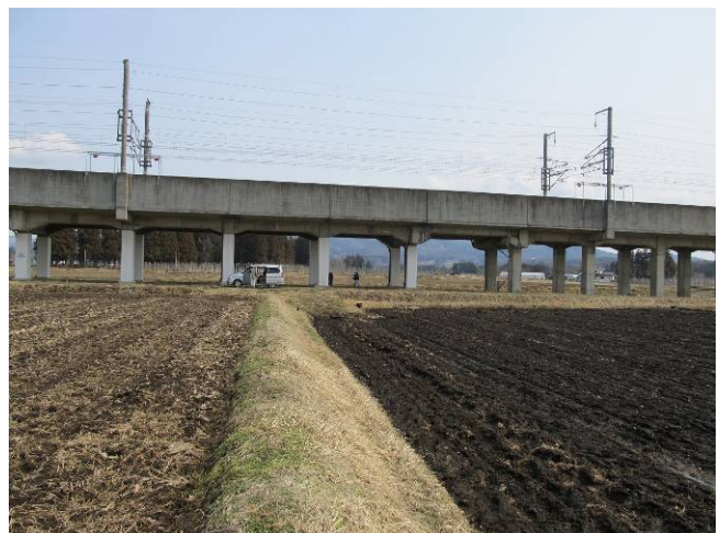
No. 5 Inohana BL R13 (Seismically retrofitted after damage)
