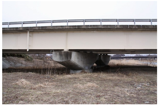
Toyosawagawa Bridge on the Tohoku Expressway: bridge pier skewed with respect to the bridge centerline
