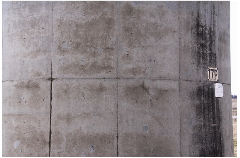
No. 1 Kitakamigawa Bridge 17P: Minor cracks (Closeup of the photo to the left)
