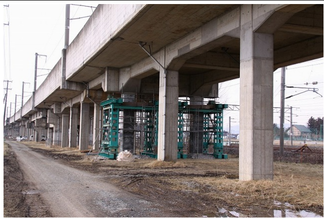
No. 1 Akabayashi BL R2 (columns at both ends): damaged (and repaired) (The nearer rigid frame in the photo is R2.) Emergency repair work was being carried out on the two columns at the Tokyo end and one column at the Morioka end. No noticeable damage was observed on intermediate columns, although flexural cracking was seen.
