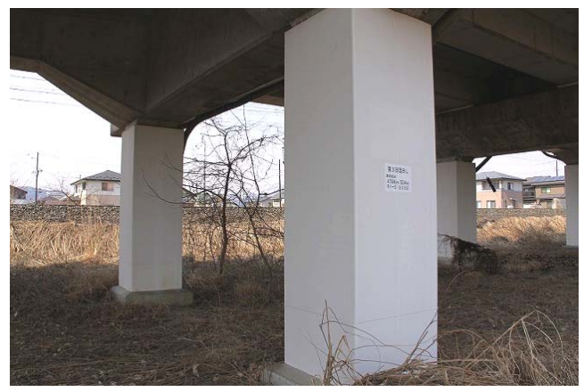
No. 3 Hizume BL R1 side columns Columns had already undergone seismic retrofitting with steel jacketing.
