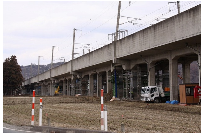
Tilted catenary poles
