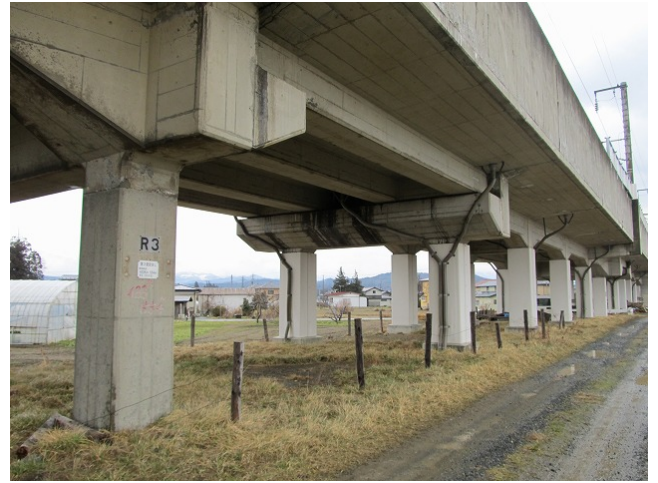
No. 3 Odagi BL R1 and R2 (Seismically retrofitted after damage): undamaged
