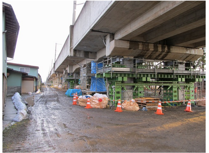
No. 1 Nakasone BL R7 North-end columns: damaged (and repaired)
