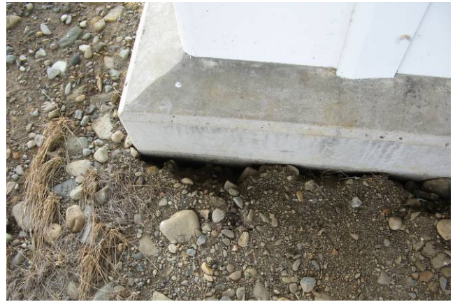
No. 5 Inohana BL R13: gap between column base and fill
