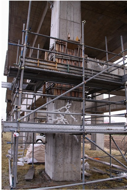
No. 2 Yachi BL R3 North-end column: damaged (and repaired) Joint: repaired by restoring the reduced cross-sectional area with grouting of the cracks 2-story column: cracks grouted with resin
