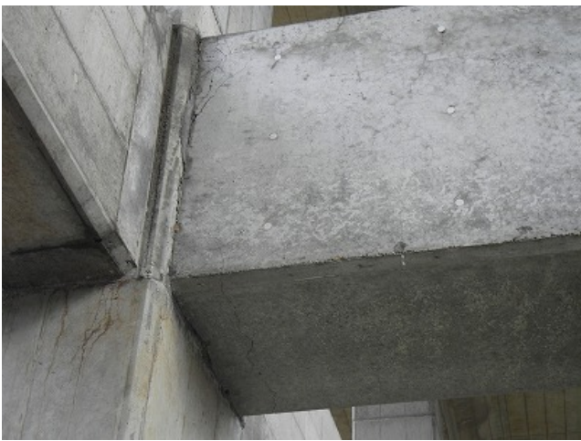
No. 2 Yachi BL R1 beam-column joint between 1 st -story column and transverse beam: flexural cracking
