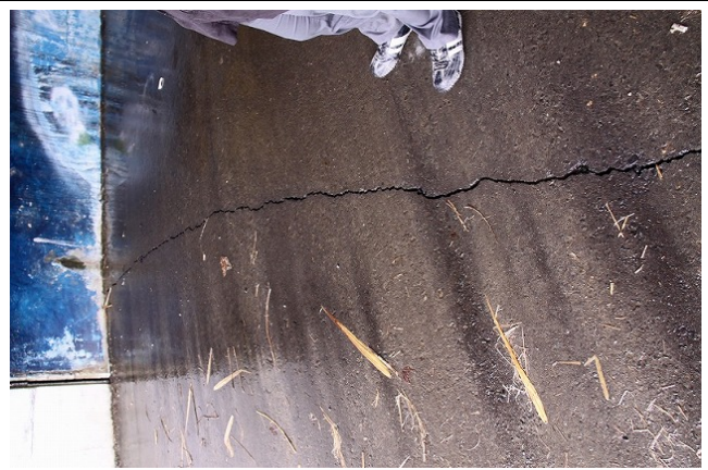
Cracked pavement in photo to the left
