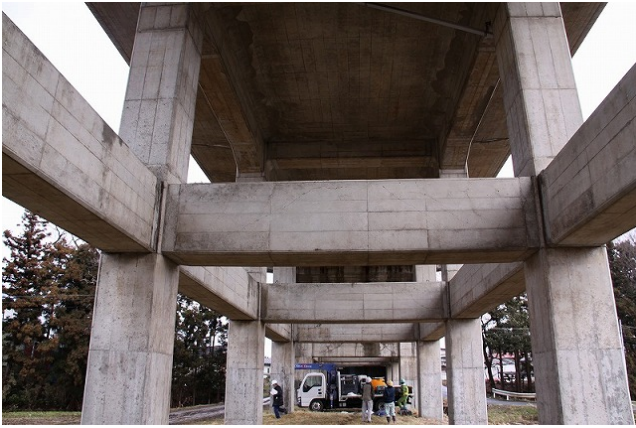
No. 2 Yachi BL R2 1 st -story transverse beam: fine diagonal cracking
