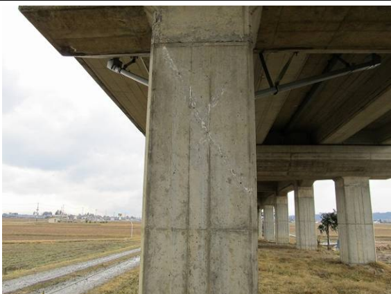
R3: Traces of cracks repaired by grouting were cracked.
