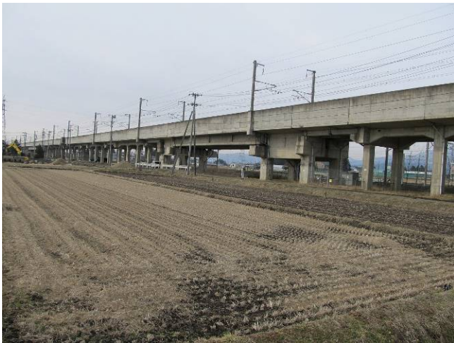
No. 1 Akabayashi BL R1 and preceding rigid frames: undamaged
