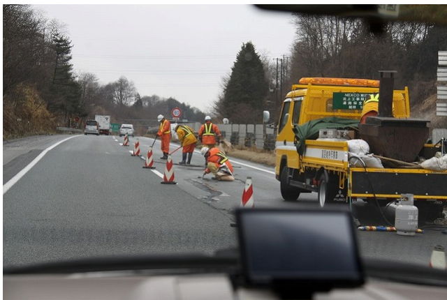
Cracked pavement (minor damage)
