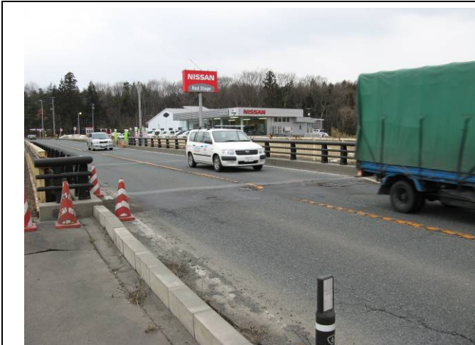
Iide Bridge on National Road No. 4 The fill behind the abutment settled, causing a difference in road level.
