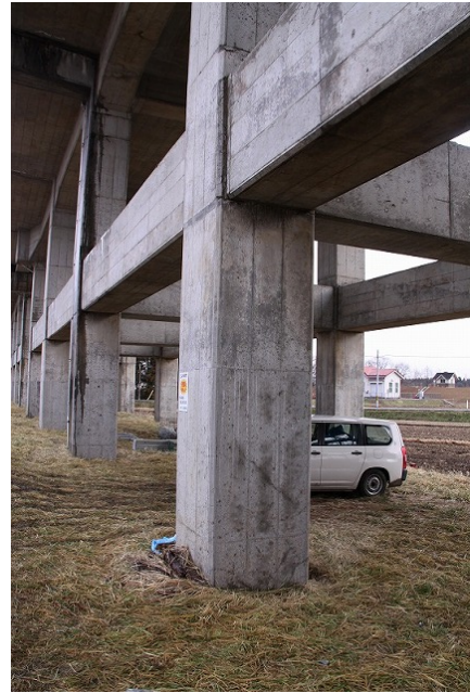
No. 2 Yachi BL R3 intermediate column at North-end: cracks found Diagonal cracks developed on the surface of the intermediate column in the longitudinal direction.
