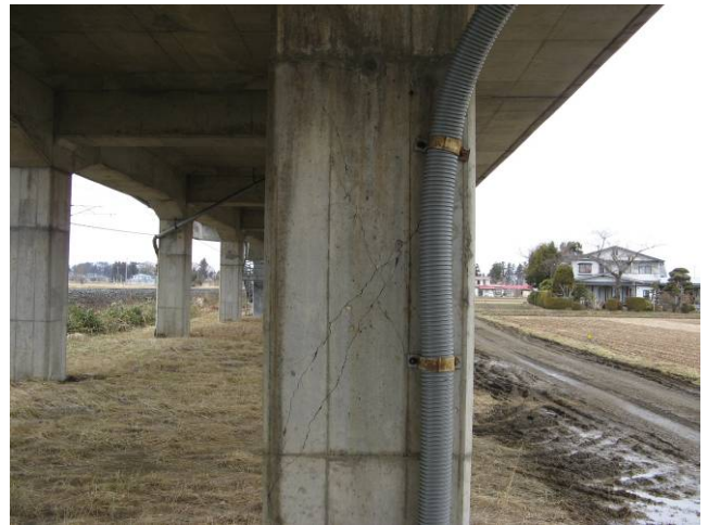
No. 3 Tokuta BL R1 intermediate column: cracks were observed (not yet repaired) X-shaped diagonal cracks were found on the column surface facing the longitudinal direction
