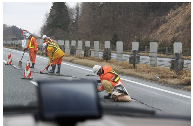
Cracked pavement (minor damage)
