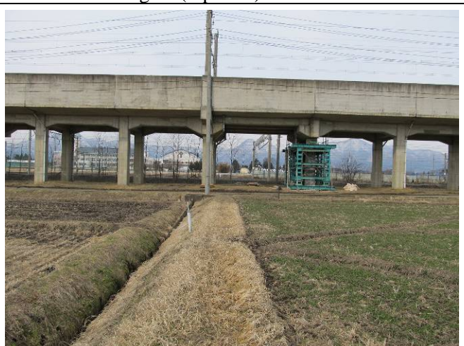
No. 1 Akabayashi BL R1: undamaged R2 (left column): damaged (and repaired)
