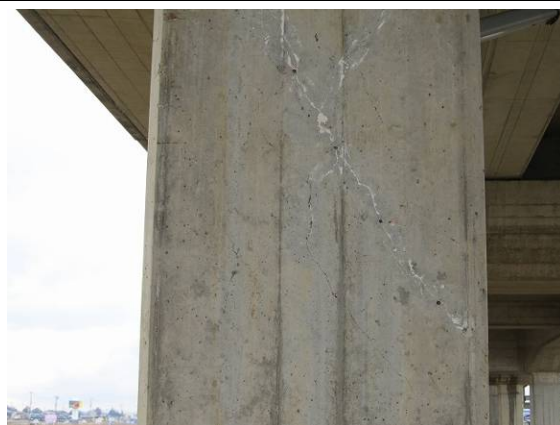
R3: Closeup of damage in photo at left
