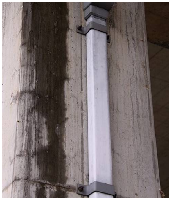
Closeup of the photo to the left Narrow diagonal cracks developed.
