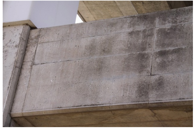
Yahaba Minami BL R1 to R5 (closeup of the 1 st -story beam end in photo to the left) The 1 st -story transverse beams: fine cracks were found.
