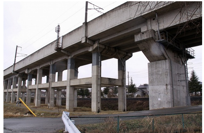
Yahaba Minami BL From the right: Ainono BV P1, R11 to R10 No noticeable damage was found in columns, although shear cracking had occurred in the 1 st story transverse beams.
