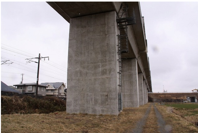
No. 1 Minami Yahaba BL 12P and subsequent piers: undamaged Bridge piers had already undergone seismic retrofitted by the RC jacketing method. (Thickness of RC jacketing unknown)
