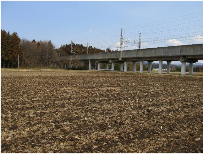
No. 5 Inohana BL R14 (Seismically retrofitted after damage)
