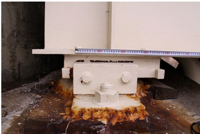
Toyosawagawa Bridge on the Tohoku Expressway: support point moved due to earthquake
