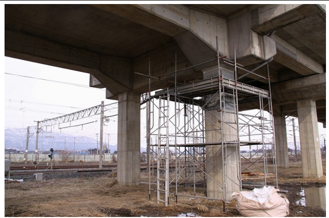
No. 1 Akabayashi BL R2 north end columns: damaged (and repaired) Of the R2 bridge pier columns at the north, only the right column (on the near side of this photo) was being repaired. R3 on the far side in this photo was undamaged.
