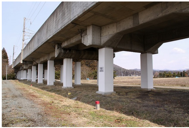
No. 5 Inohana BL R13 in foreground and R14 behind: no damage to main structural members Columns had already undergone seismic retrofitting with steel jacketing.
