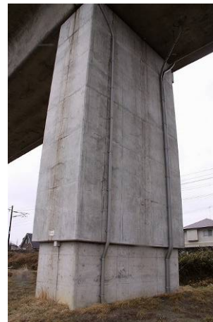
No. 1 Minami Yahaba BL 8P: undamaged The bridge pier had already undergone seismic retrofitting by the RC jacketing method. (Thickness of RC jacket: 20 cm)
