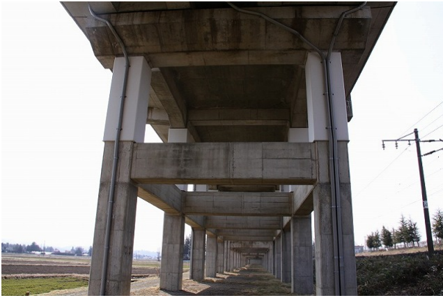
Yahaba Minami BL R1 to R5 (2-story rigid frame; the 2-story columns had undergone seismic retrofitting with steel jacketing) The 1 st -story transverse beams: fine cracks were found.
