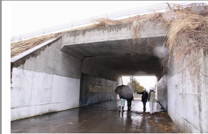
Farm road passing under Prefectural Road No. 205 The culvert was displaced and the pavement had cracked.
