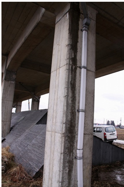
Details of longitudinal-facing surface of damaged intermediate column Narrow diagonal cracks developed.
