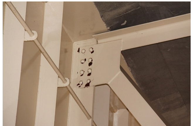
Toyosawagawa Bridge on the Tohoku Expressway: peeled paint film on a gusset plate above the support point on the bridge pier.
