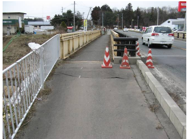
Iide Bridge on National Road No. 4 The fill behind the abutment settled, causing a difference in road level.
