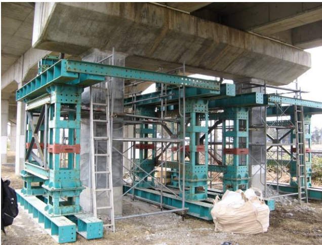
No. 3 Tokuta BL R1 columns at the South end: damaged (and repaired)
