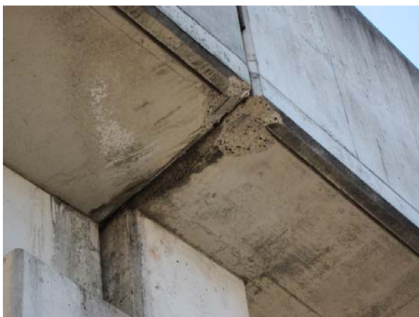
Fig. 1.3 Damaged cantilever girder
