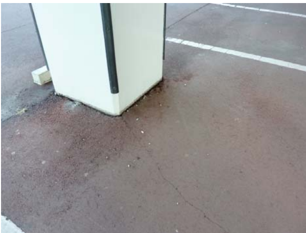
Fig. 3.2 Cracking at the column base of rigid frame viaduct
