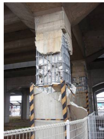
Fig. 1 Details of damage to the Naka Nagamachi viaduct (Source: East Japan Railway Company)
