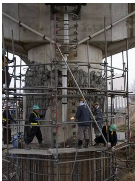
Fig. 1 Details of damage to bridge pier 4P of Iwakiri viaduct (Source: East Japan Railway Company)
