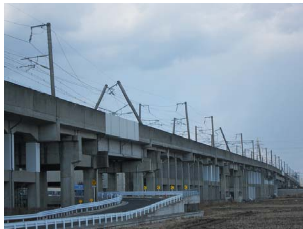
Fig. 1 Damaged catenary support poles on the Tohoku Shinkansen line
