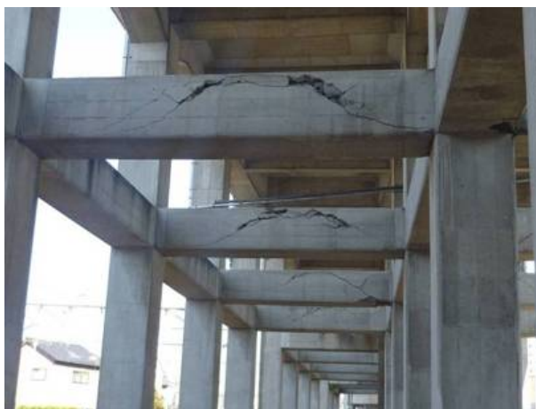
Fig. 1 Details of damage to block R1 (Source: East Japan Railway Company)
