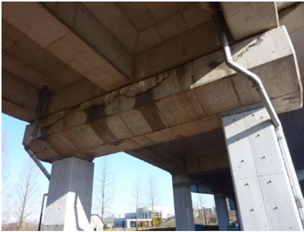
Fig. 2 Damaged girder support
