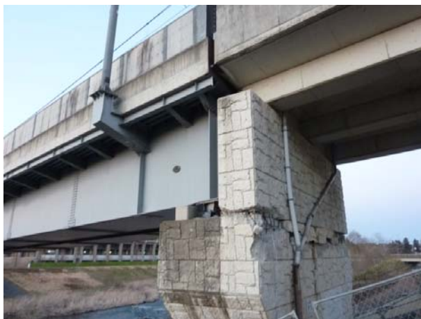
Fig. 1.1 General view of damaged breast wall
