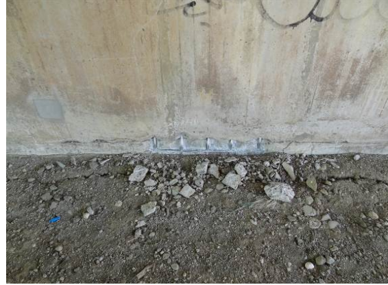
Fig. 4 (Closeup of the damaged portion in Fig. 3)
