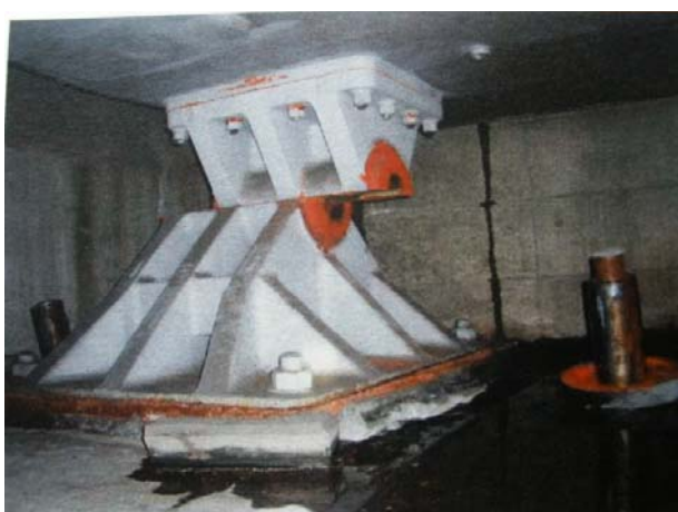
Fig. 2 Details of damage to bearing (Source: East Japan Railway Company)
