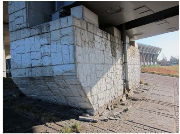
Fig. 3.1 Deformed ground (Nanakitagawa bridge, Izumi Chuogawa abutment)
