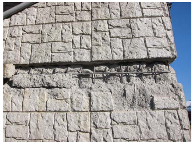
Fig. 1.2 Details of damage to the breast wall
