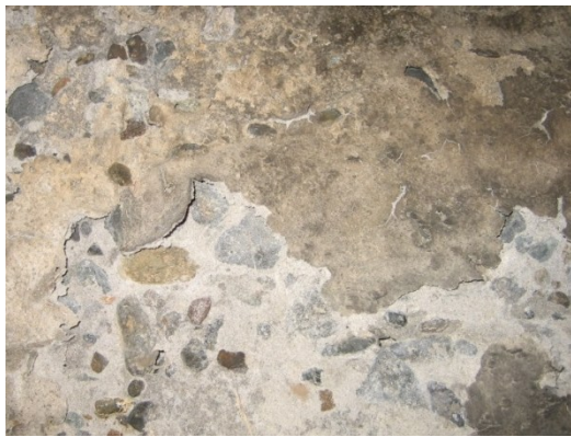
Photo 1. Deterioration of tunnel lining concrete
