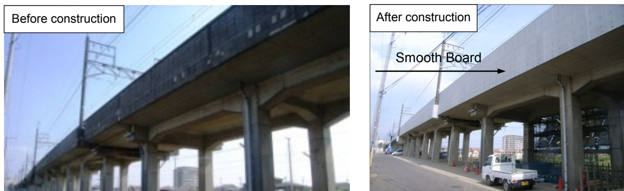
Photo 8. Repair of railway viaduct side wall (1.6 m high before construction; 2.5 m after rehabilitation)
