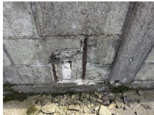
Photo 2. Deterioration of railway side wall (reinforcing steel is corroded and exposed)
