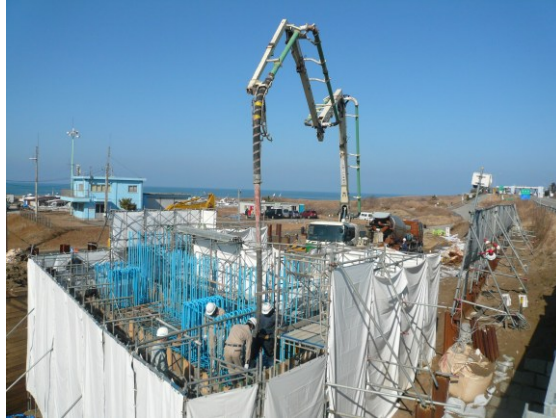
Photo 2. Construction of fly-ash concrete abutments on a local road in Ishikawa prefecture.
