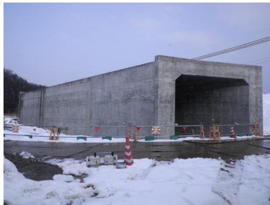
Photo 3. Completed fly ash concrete box culvert on a national road in Ishikawa Prefecture.
