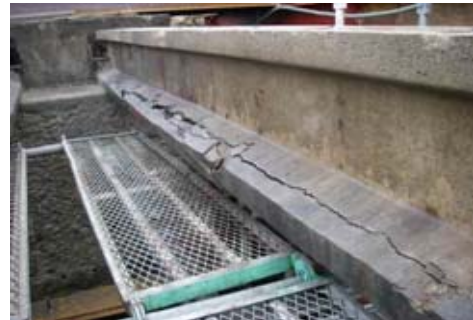
Figure 1: Deteriorated PC girder (beam D)
