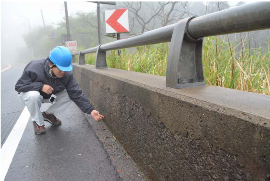
Photo 5 Deterioration of safety barrier due to freezing damage
