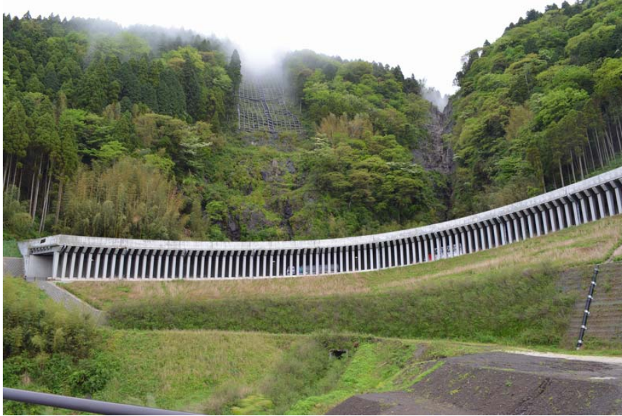
Photo 2 Rock shed and slope protection structures near to the beginning of the Takimurozaka section
