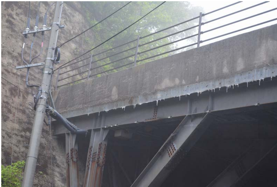
Photo 6 Deterioration at entrance to rock shed, middle of Takimurozaka section
