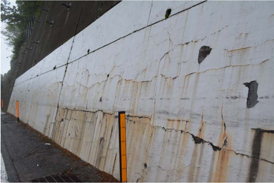
Photo 4 Deterioration of retaining wall possibly due to ASR
