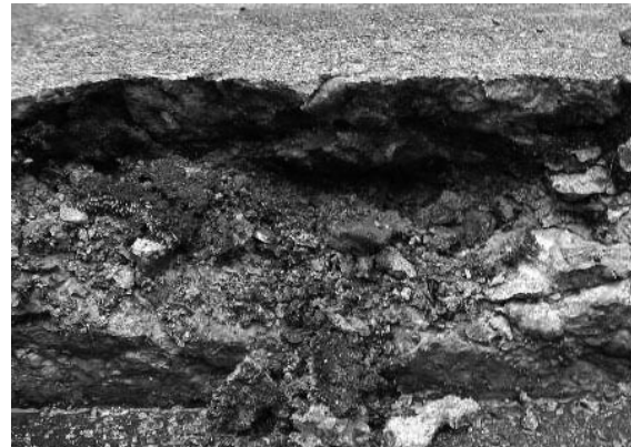
Photo 2 Severe scaling of wheel guard concrete
