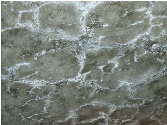
Photo 1 Mesh-pattern cracks and white deposits on under surface of bridge deck
