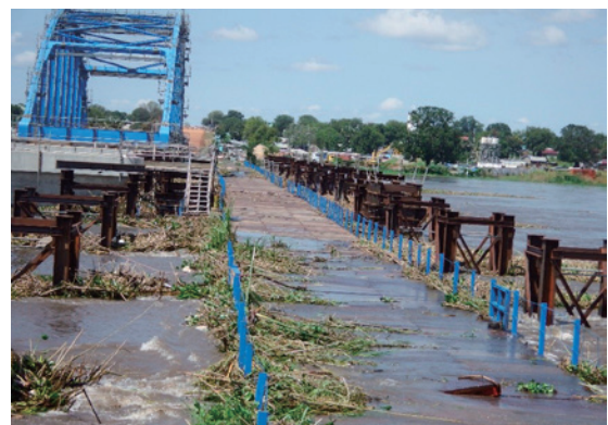
Photo 9: Water Level Overflowed Temporary Bridge
