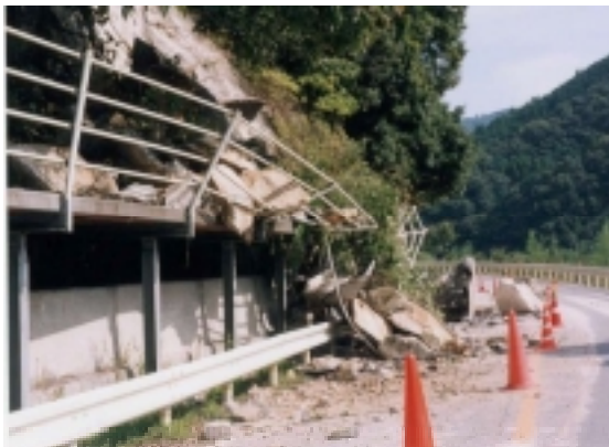
Earthquake Damages in Tottori Prefecture
